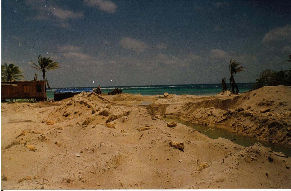
Picture B. Inshore trench where the water intake-pipe was deployed. The close proximity to the sea and the amount of sediments being accumulated are clearly visible.
